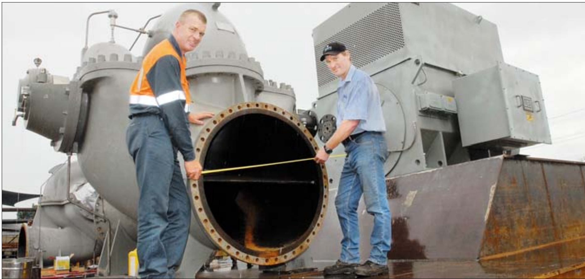
MACS Engineering project manager Allan Brett, left, and director of engineering Shane McNeilly with Australia's biggest pump.
